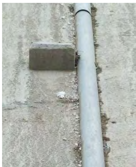
d) Concrete block and cable protections.
